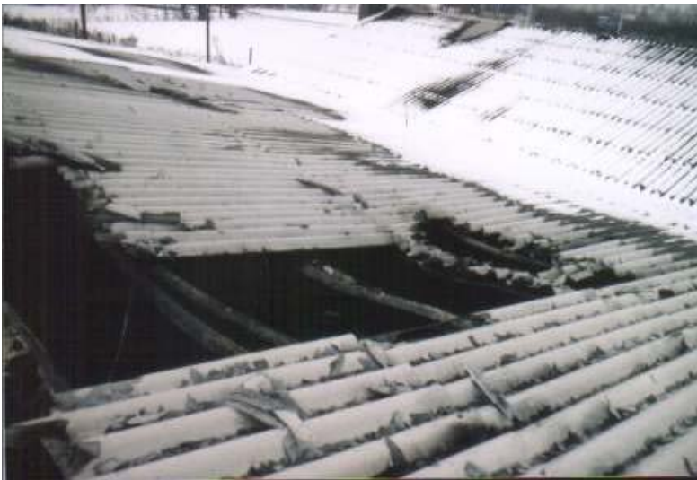
The damaged roof of Hall 6 from the fire in 1980.
